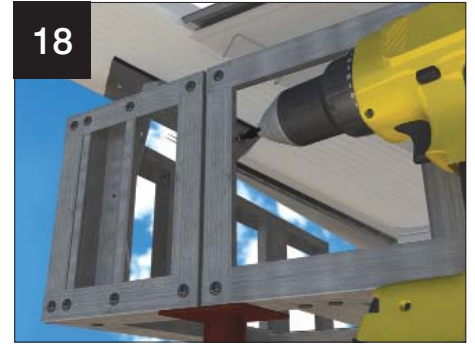
18 Fit the vertical frames. Fix the frames into the valley corner infill and the horizontal frames.
