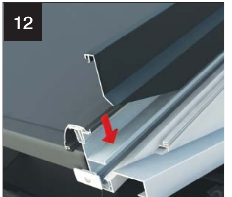
12 Scribe and cut the bottom end of the cloaking trim horizontally for a flush fit on the gable beam.
