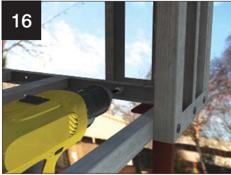
16 Fit the valley corner infill panel to the horizontal frame, level up and secure to the valley plate.
