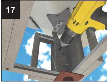
17 FIT THE STRAP CHA018 USING M4x13 SELF DRILL SCREWS, to the valley corner infill panel and the valley fixing bracket. It may be necessary to bend CHA008 to suit.
