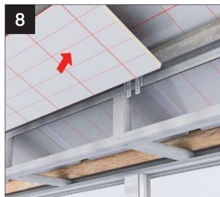
8 Next fit the 25mm insulation board, which is 590 x 2400mm. These boards must be laid at right angles to the glazing bars and run across the bars.
