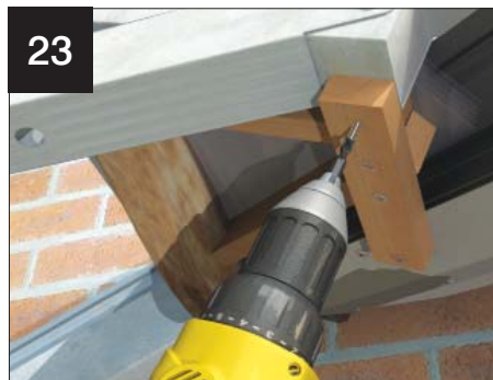
23 Fix into position using plasterboard screws. NOTE: when fitted, the battens should terminate at the centreline of the steel undercladding to allow for fitting of the adjacent panels
